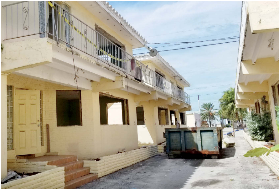
In this “before” photo, the debris is gone but reconstruction has not started. Below: a new thrift shop facing the Overseas Highway. St. Columba photos
