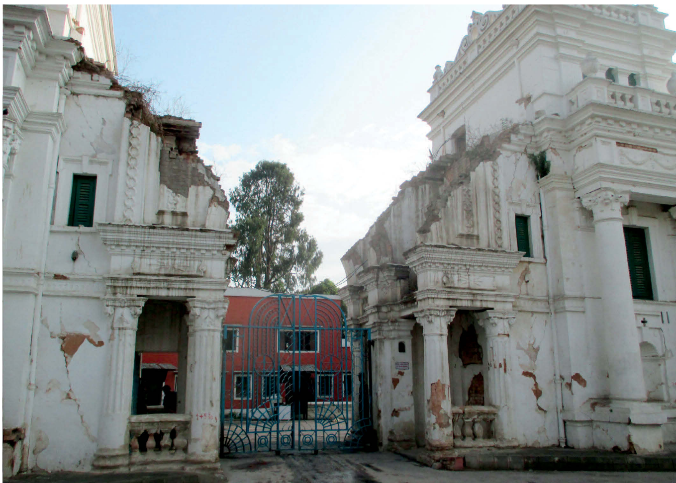
The badly damaged entrance to the former royal palace
