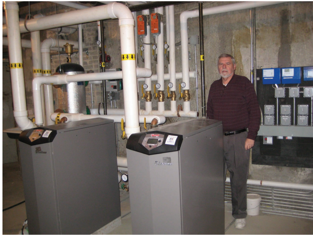
The complete heating system at Trinity Church
