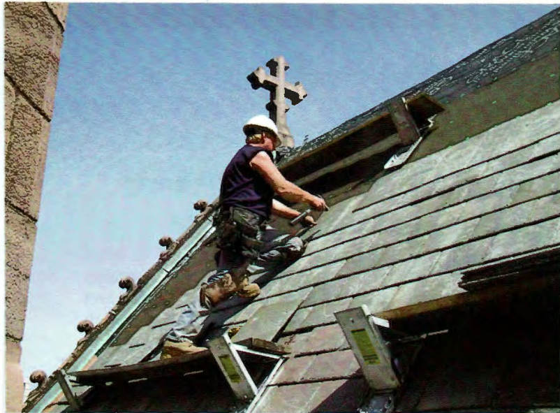
A new slate roof was installed recently at St. Paul's Cathedral, Buffalo, N.Y.
