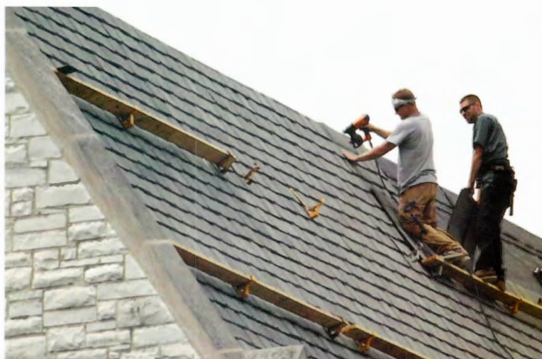
After 50 years, a new roof for Christ Church, Whitefish Bay, Wis. Rick Wood photo
