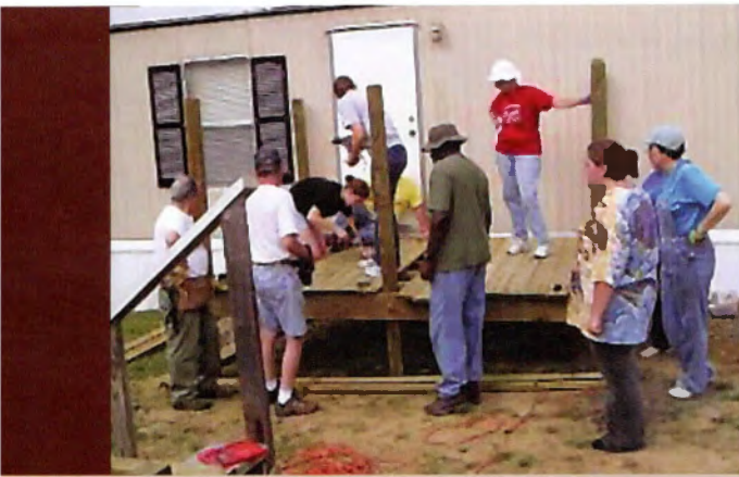
The team from Emmanuel, Hampton, Va., builds decks on trailers used as temporary housing for families affected by flooding in West Virginia.
