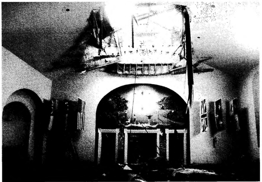
The force of the wind caused the church bell to fall through the roof of Christ Church, Pensacola, Fla.
