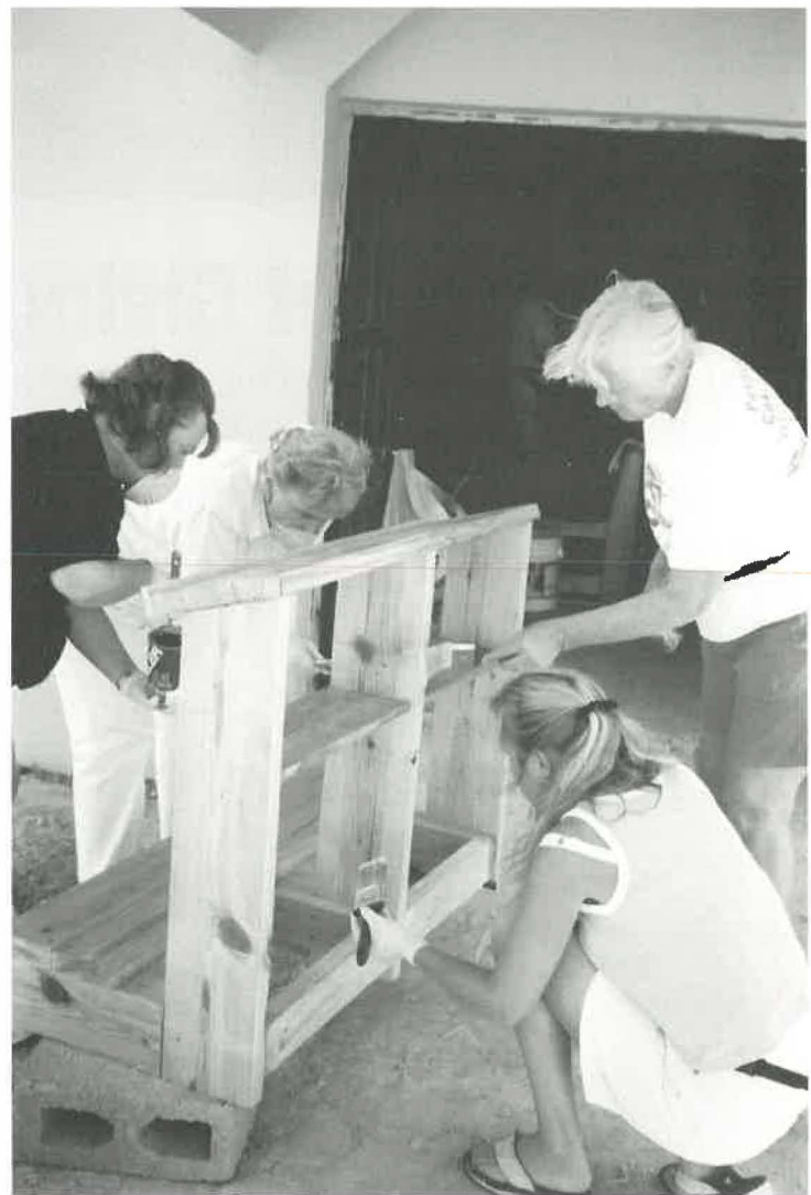
Workers painting the red trim on the cross (left) and finishing a prayer bench (above). Chuck Miller photos
