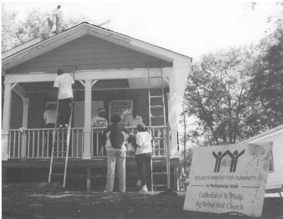
St. Philip's and Big Bethel AME Church members build a house for Habitat for Humanity.
