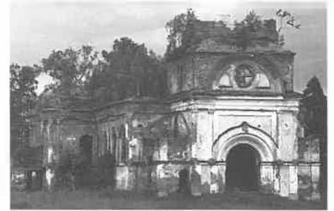
ABOVE: The cupolas, doors and windows are gone, but much of the Church of the Dormition has stayed intact.
