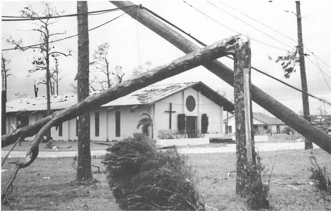
The hurricane tore up the roof of Church of the Ascension, Richmond Heights, south Dade County.
