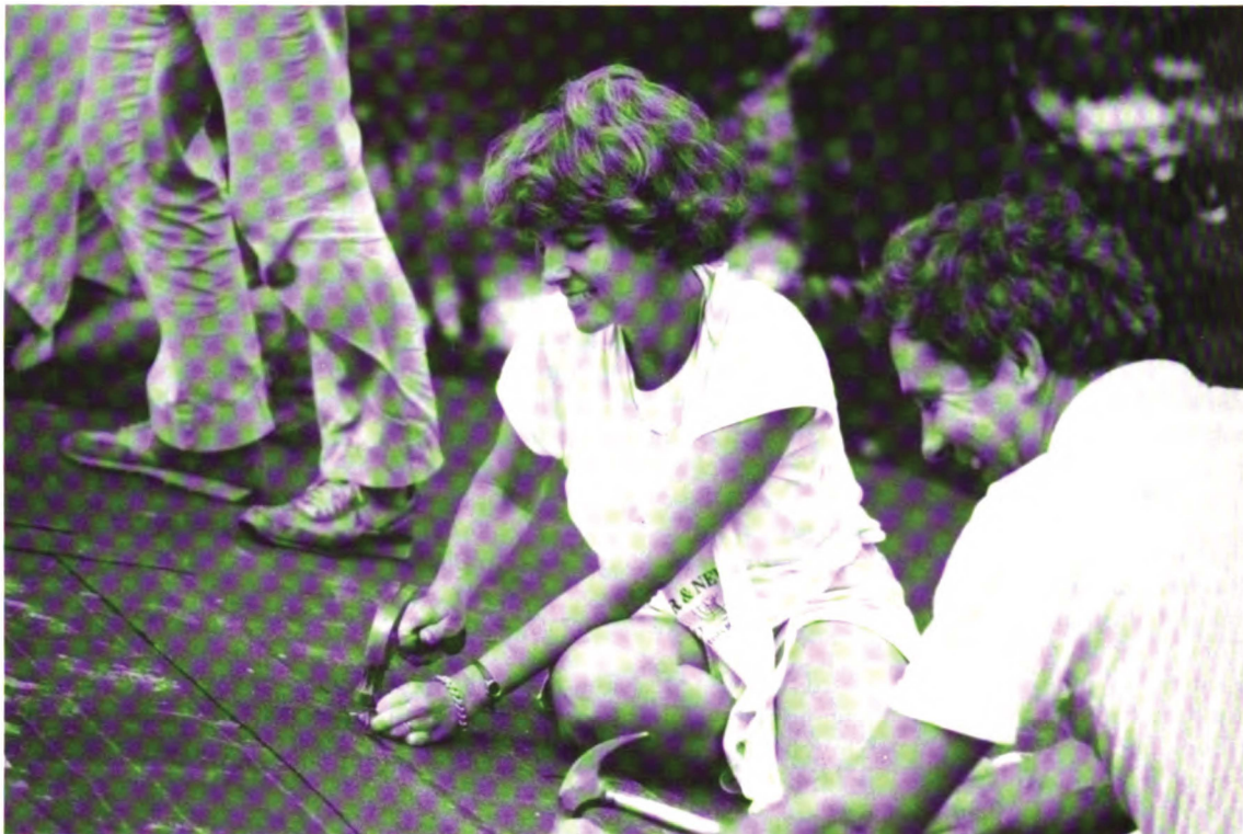
Dottie Schipper and Jan Williams of Christ Church work on a Habitat for Humanity house in Greenville, S.C.
