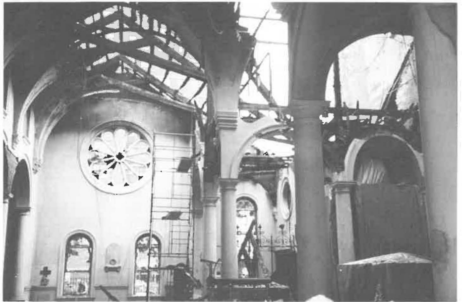
Burned timbers are all that remain of much of Holy Apostles' roof. [ENS photo by Jeffrey Penn.]
