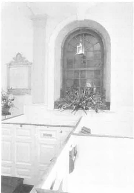
A walled-over window found during restoration of Old North Church in Boston has been confirmed as the escape route for church sexton Robert Newman after he signalled with lanterns to warn the patriots of the British advancement and begin the ride of Paul Revere. [RNS]
