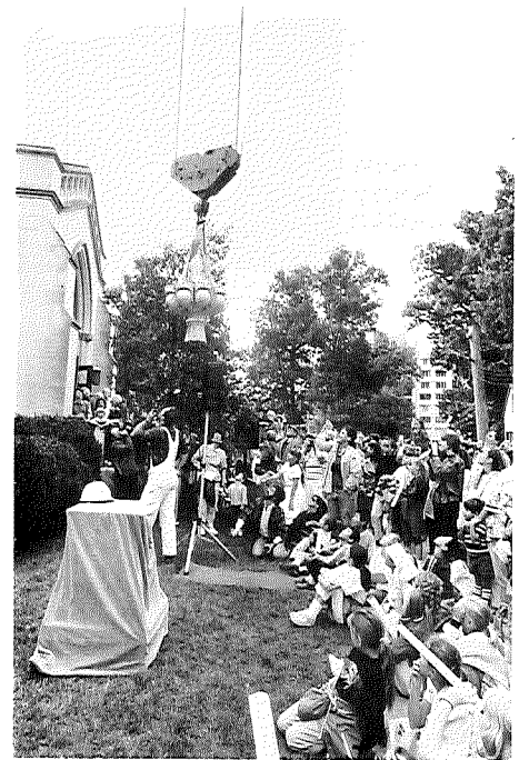
A crane raises the national cathedral's capstone to be set in place: "a house of prayer for all people."
