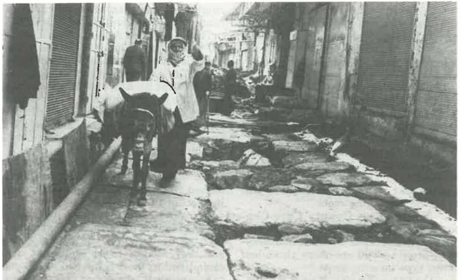
An Arab leads his donkey over large paving stones that are believed to be part of a road that dates back to 500 A. D. Located in the Christian quarter of the Old City of Jerusalem, the stones were uncovered during work on a new sewage system.
