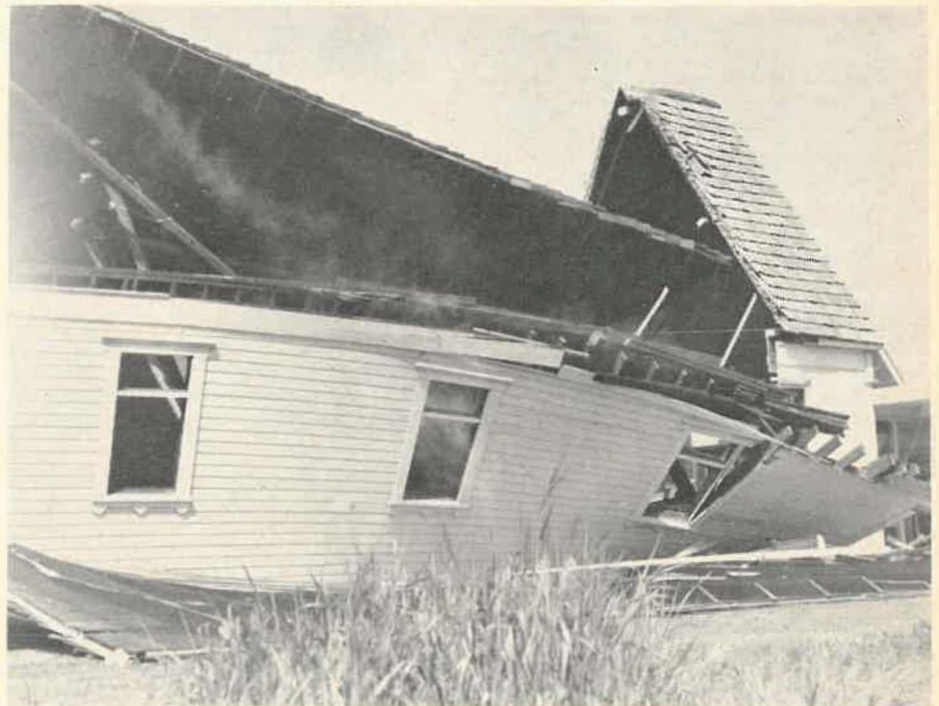
St. Matthew's Church, Auburn, Wash., was declared unsafe by city officials after the sharp earthquake which rattled through the Puget Sound area of western Washington on April 29th. The church, built in 1895, had been moved in 1958 from its original location across from the Auburn City Hall. Under the direction of the Rev. Alfred A. Cramer,
