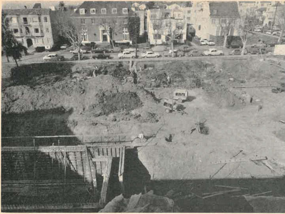
This hole in the ground is certainly "not a thing of great beauty," as Garret Conklin, vice-dean of the Church Divinity School of the Pacific, Berkeley, Calif., comments, but it is "the newest thing that is happening at CDSP." From this hole is steadily rising a new million-dollar dormitory-refectory-lecture-room complex.
