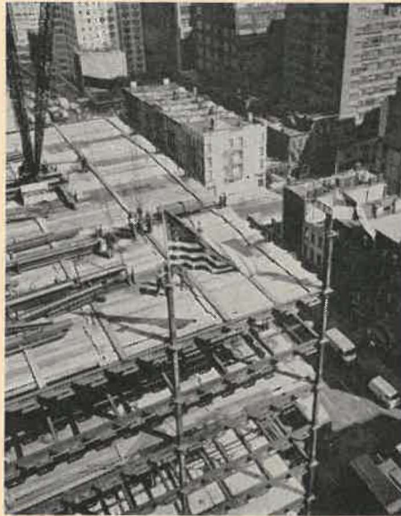
Side by side over Manhattan wave the flags of the United States and the Episcopal Church, as the new Episcopal Church Center in New York City is "topped out." The flags mean that steel for the topmost of the 12 stories in the building has been set in place. According to the Bethlehem Steel Co., suppliers for the job, the center is the first building in Manhattan to use a new high-strength, low-weight steel frame which received New York City's approval only last year.
