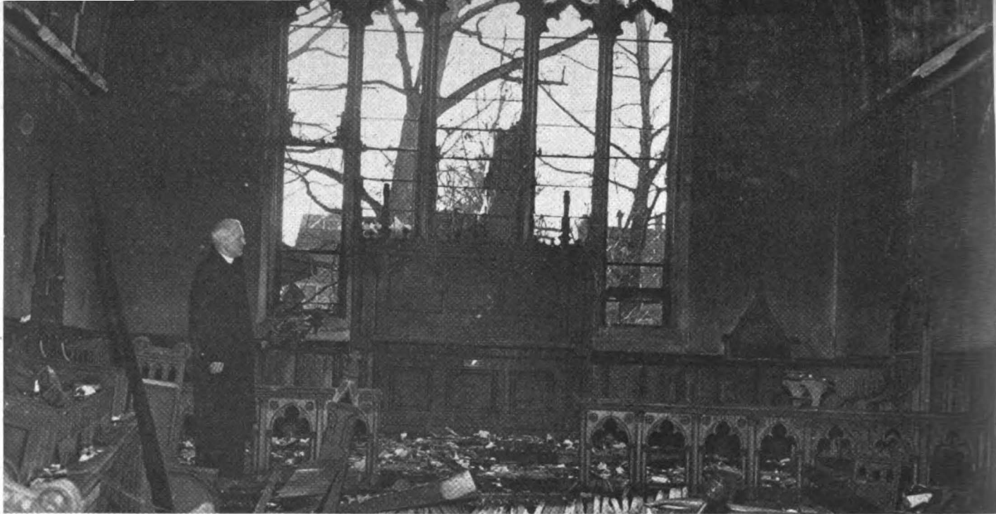
The wide-open areas of the church give a fire plenty of breathing room. [Cut is of Church of Good Shepherd, Shelton, Conn., with rector, the Rev. Fred P. Sutton, viewing ruins of 1957 fire.]
