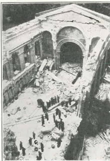
Acme Radiophoto. GUARDS CHAPEL: Many casualties resulted when this noted London church was demolished by robot bombs during a service [L. C., July 16th].
